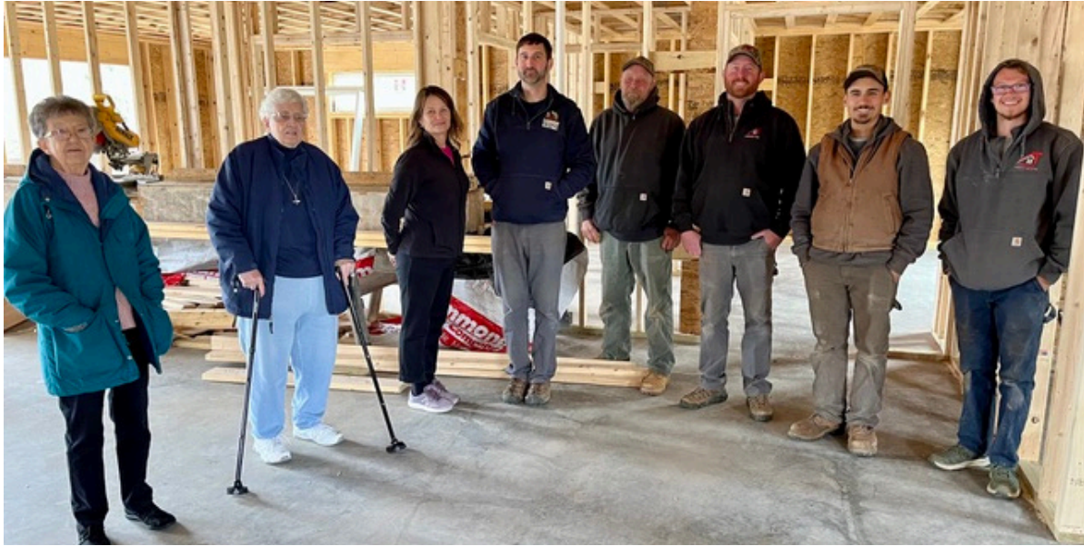
(L to R): Srs Claudette and Janet, with Marcia our Community Support Coordinator, Justin Lambert our electrician, and General Contractor Zak Foote and his construction crew, review the progress on turning the one-bedroom apartment adjacent to our St. Joseph Center into a two-bedroom, handicapped-accessible residence.
